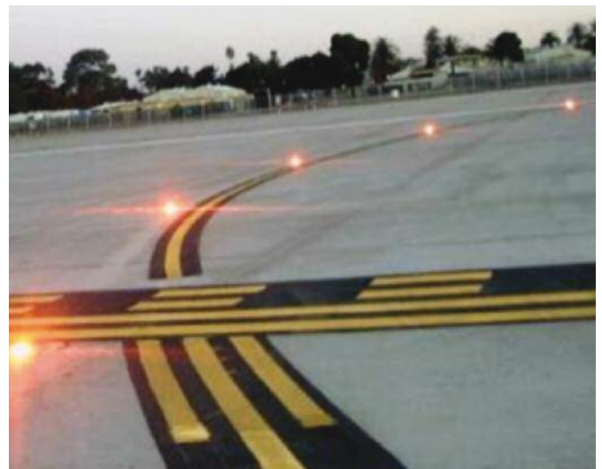
Runway Entrance Lights (RELs).
